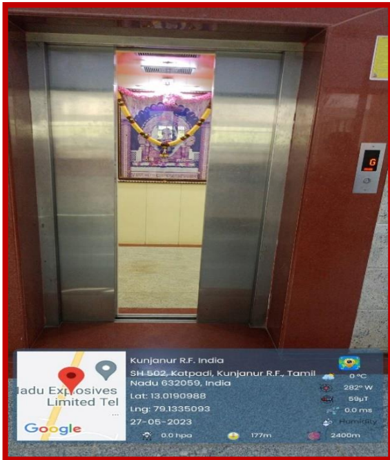
Lift in Admin Block
