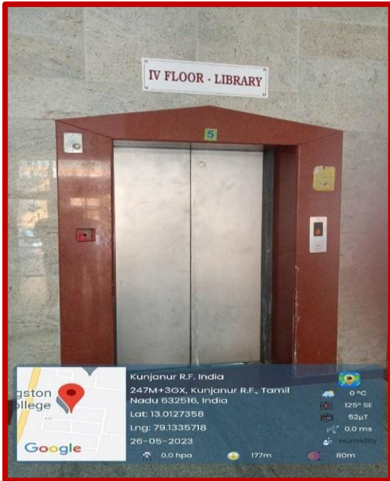
Lift in Library Block
